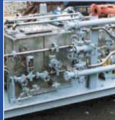
API 614 lube oil skid with Hycoa transfer valves
