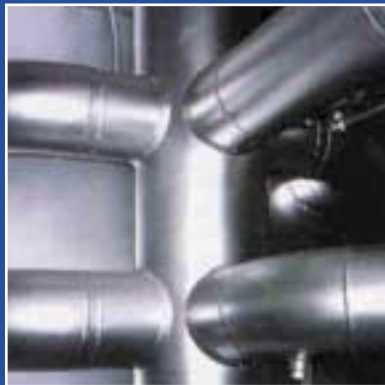
Intake lube oil transfer valve for large gas turbine manufacturer
